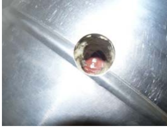
Bored Hole at the 6 O'clock position exposing bare pipe surface
