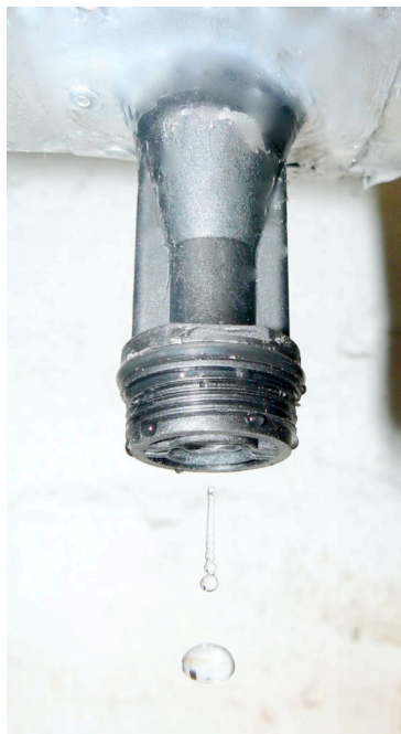
This picture clearly shows fluid exiting the collector funnel from within the insulated pipe
